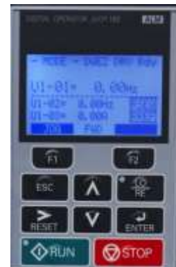
Operator's control panel
